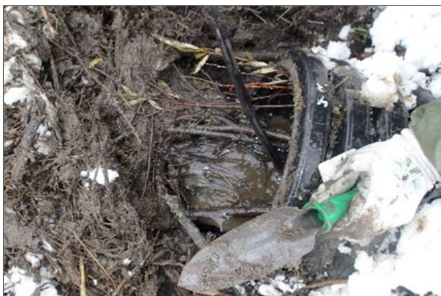
Sometimes, busier-than-normal beavers can plug the downstream end of the pond levelling pipe – a situation that is uncommon. We believe it occurred because this pipe flows into another beaver pond immediately downstream, which allowed easy access to the pipe.
