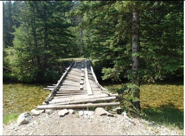
QUAD BRIDGE IN NEED OF REPAIR, UPSTREAM FROM FORDED STREAM CROSSING (Photographer: J. Melsted, Catalogue No: RHIP02GOL007)
