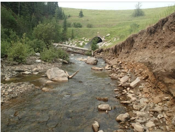
Photo g: Disturbance-caused plant communities are concentrated in many sites to disturbed road ditches, such as the Highway 40 crossing at the upstream end of VIC1 on Vicary Creek. (Photographer: J. Melsted, Catalogue No: RHIP01VIC007)
